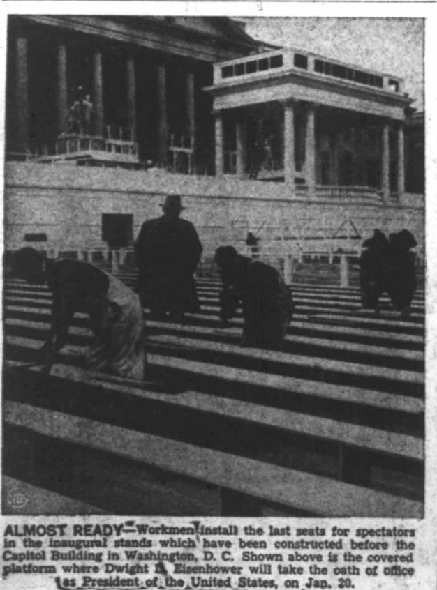
ALMOST READY—Workmen install the last seats for spectators in the inaugural stands which have been constructed before the Capitol Building in Washington, D. C. Shown above is the covered platform where Dwight D. Eisenhower will take the oath of office as President of the United States, on Jan. 20.
