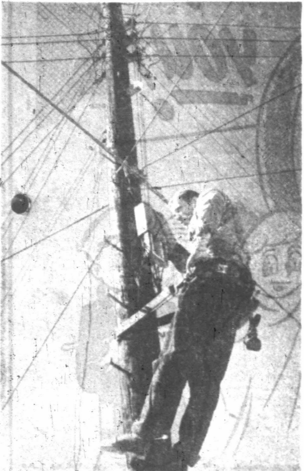
NOW WHERE DOES THIS WIRE GO? —A telephone lineman solves the cross-wire puzzle before he as Southwestern Bell Telephone Company prepares to extend its facilities to 1,700 new Midland patrons.
