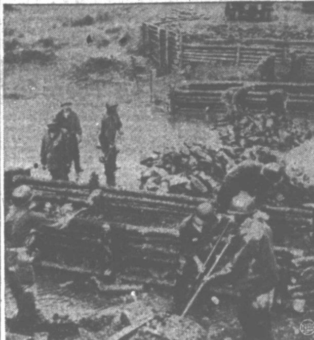
BRIDGE BUILDERS—UN engineers work ankle-deep in water to complete a new bridge over a Korean creek which will improve the supply line to Old Baldy. Defending UN troops atop the vital hill continue to throw back fanatical Red counterattacks.
