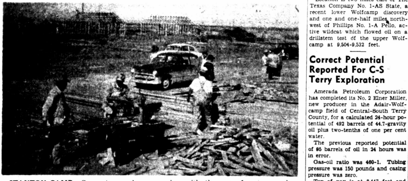
STANTON CAMP—Carpentry work progressing with the use of power equipment at the Humble Oil & Refining Company's Stanton camp. This housing is being erected by Whitmor Homebuilders, Inc.
