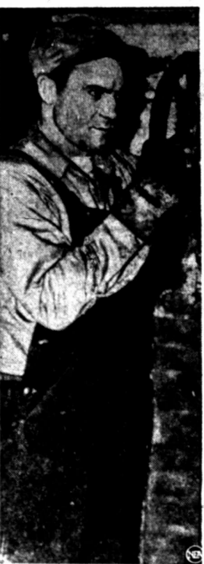
MAN AT WORK—Hank Bauer goes about his off-season job as a pipe-fitter. The Yankees' World Series star is helping install a new sprinkler system for a huge Kansas City Kan. garage, severely damaged by the Summer flood. (NEA)
