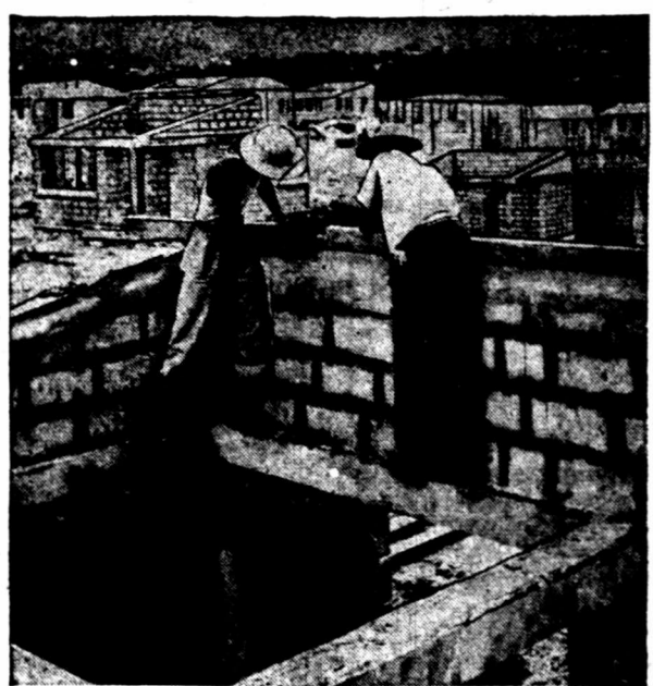
HOMES FOR HAITIANS—For the first time in the colorful history of the western hemisphere's only French-speaking republic, low-cost housing is being built for Haiti's "little man." The first "Workers' City" is nearing completion at Port-au-Prince, where these workers are seen building one of the new homes. A wide-spread social and economic reform program of President Paul Magliore calls for 15 low-cost housing projects throughout the island at a cost of about $564,000.
