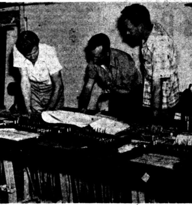
NEW TOLL BOARDS —Technicians of the Western Electric Company are shown installing new long distance toll boards at the Midland office of Southwestern Bell Telephone Company. These complicated mechanisms are being installed by, left to right, James R. Rapier, John Pugh and Jack Weir.
