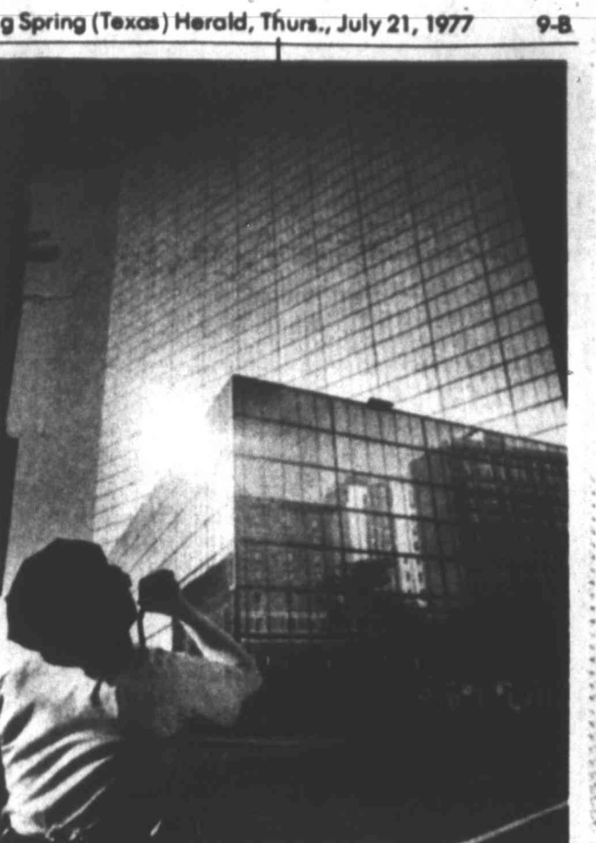
VIGIL OVER HANCOCK'S PANE - Security guard keeps his eyes peeled for cracked glass at Boston's 60-story John Hancock Tower Wednesday. All 10,344 panes were replaced with stronger glass two years ago, but they still crack and fall out. Now guards will spot cracks by change in color, yell to clear the streets, then alert technicians to reverse the air-conditioning fans to create a slight sucking force that will make the faulty glass fall inward.
