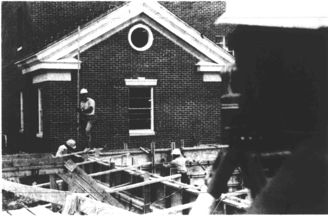
"THE LAY OF THE LAND" — Surveyors at the First Methodist Church take measurements for the half million dollar construction project. Rodman at the left is Kevan Amonett, while Josh Beebe lines up his sights.
