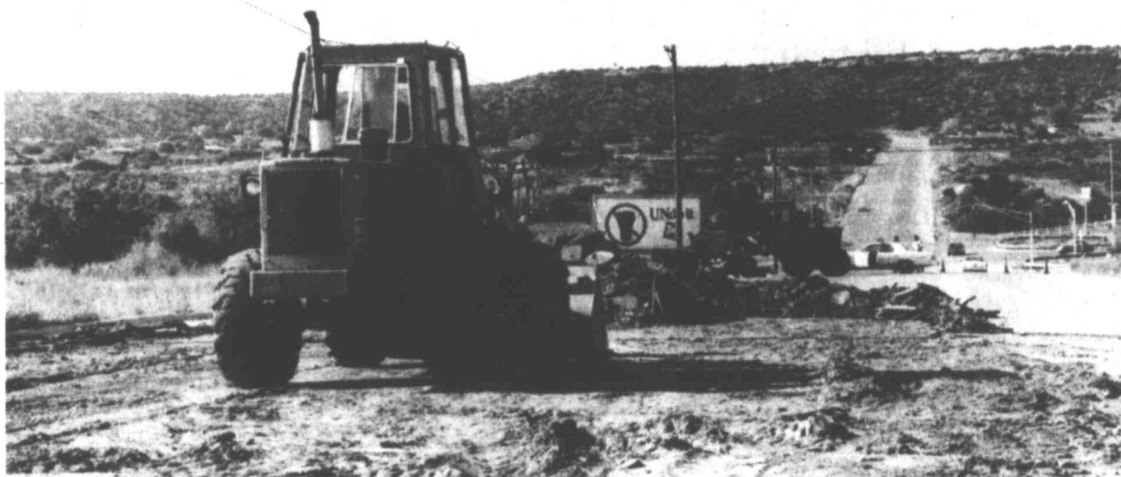
BROKEN MAIN — The pavement was floating when a 12-inch water main broke, spilling over 100,000 gallons of water beneath Goliad, according to D.W. Overman, water district supervisor. The leak was repaired Tuesday night,
