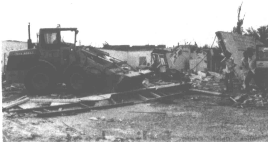
BULLDOZERS — Some of the homes in Monahans are past repair and bulldozers were cleaning up the debris. R.M. Oliver of Big Spring was in Monahans helping salvage bolts of materials and other items at his sister's Fabric Shop.
