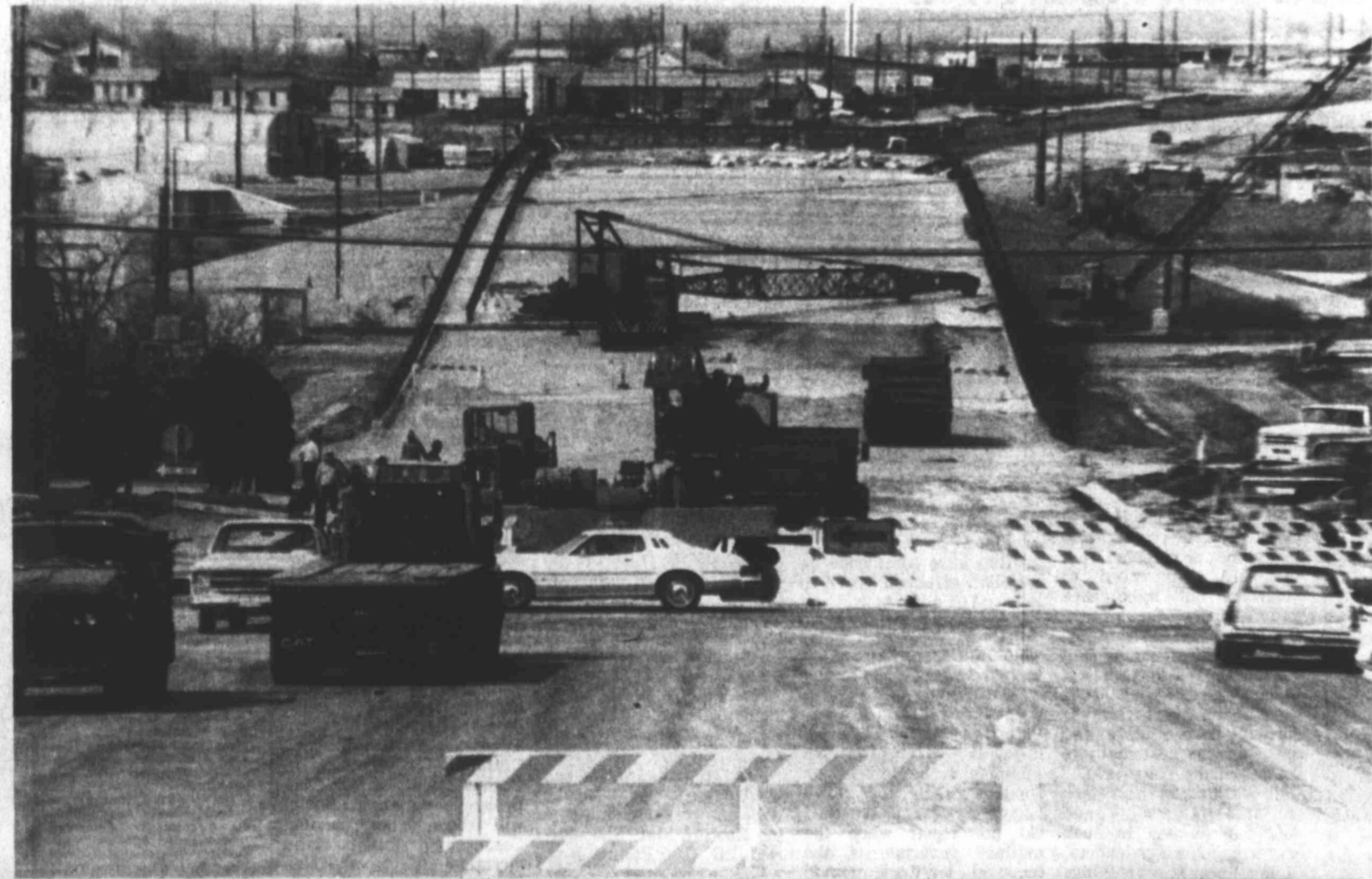
COMING ACROSS — The overpass at Owens is coming across with Owens paved last week between 3rd and 4th Streets. When completed in the fall, the
