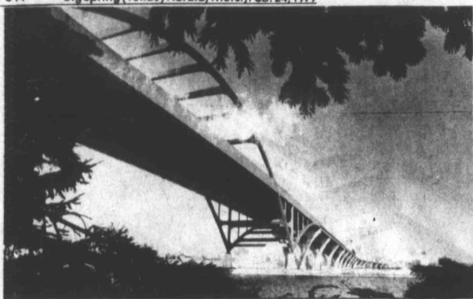
THE BRIDGE TO NOWHERE — Residents of Milwaukee have nicknamed a $75 million bridge over the city's harbor, the bride to nowhere. The six-lane structure has yet to carry its first vehicular traffic across but officials said Wednesday that the bridge should open to vehicles next fall using a partly completed ramp system connecting with existing streets. The main span of the bridge was completed in 1975 but work was stopped on freeways at both ends as a result of environmental questions raised by freeway opponents.
