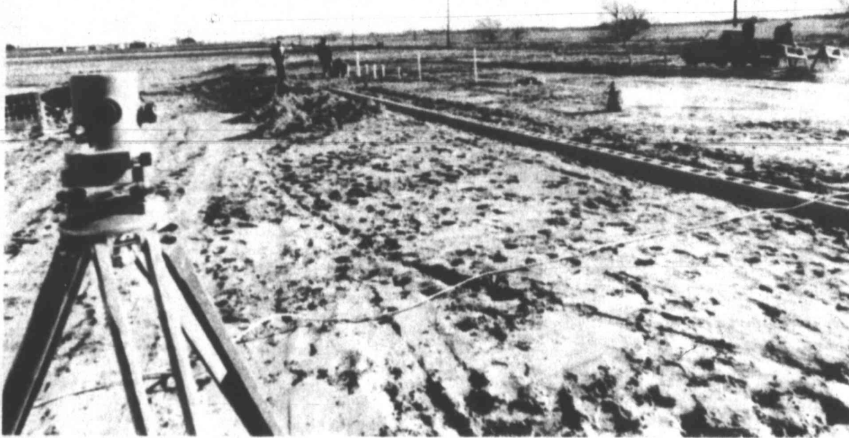
ADDITION TO PRICE CONSTRUCTION COMING OUT OF GROUND — Price Construction Company, located on the Snyder Highway, is expanding its facilities with the addition of an office building, reflecting management's faith in the Howard County economy.
