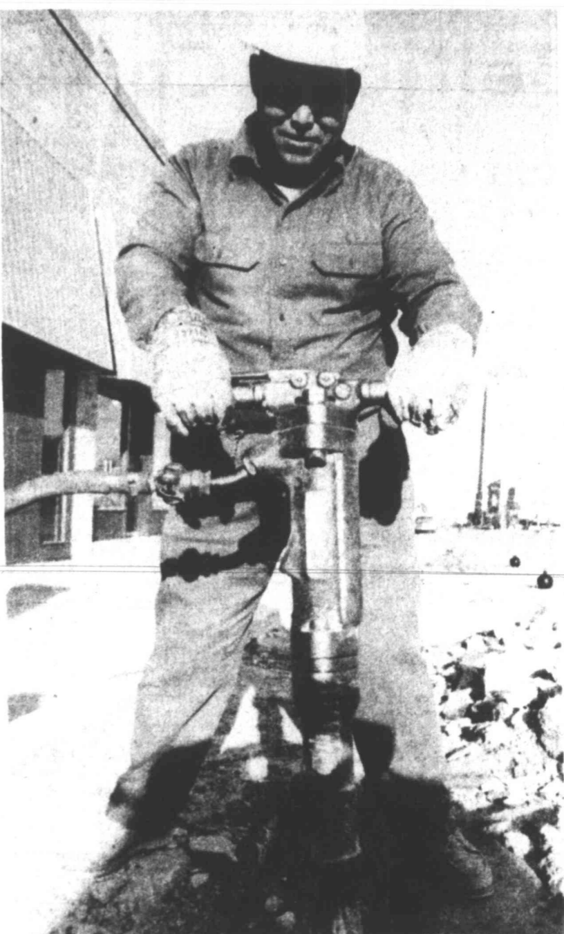
STEEL DRIVING MAN? — Jesus Alvarez, city employe, plays modern day John Henry, replacing a pick and hammer with a pneumatic drill to get to a broken water main on Third. After the main is uncovered and repaired, concrete will be used to fix the street.
