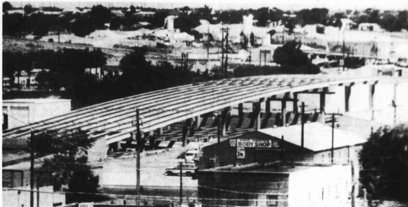
COMING ALONG — The overpass on Owens Street is showing a lot of progress. However, work will slow down as J. H. Strain Construction Co.
