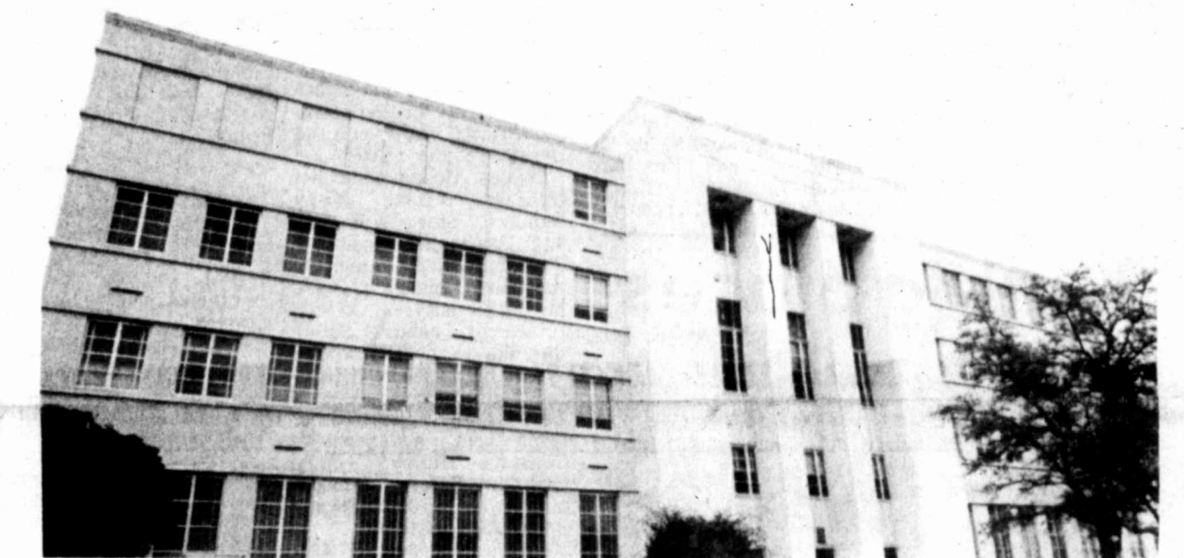
CRACKED UNDER PRESSURE? — Has the weight of years, coupled with added stress from the recent throng of local citizens entering its portals, weakened the structure of the Howard County Courthouse? Can a noticeable crack be discerned near the top of the engraving? Can the tilted building be seen in the left of the photo? Did commissioners, when contacted this morning, estimate repairs and reconstruction costs at $18.3 million? (See story on page 2, col. 5)
