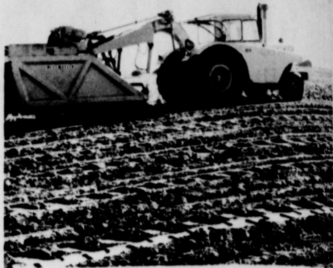
parallel terrace construction on Anna Cooper and Dick Hindengardt farm. Terraces are not the same anymore. These terraces were constructed from the back side so there would not be any channel. Also they are straight. Stop by and look at these terraces located just southeast of Gruver.
