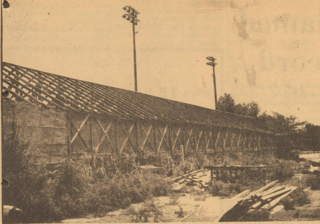
OLD LANDMARK REMOVED---The roof on the old Friona School Bus Barn has already been removed and soon the entire building will disappear from sight.
