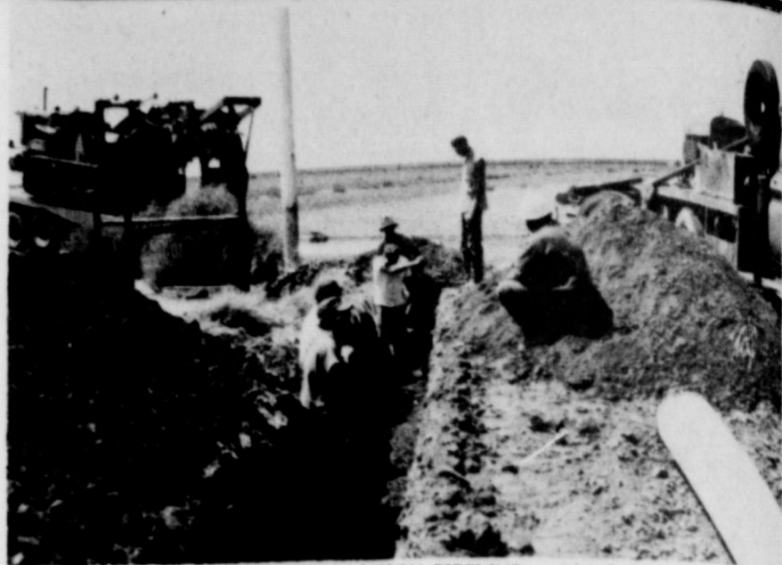
INSTALLATION OF IRRIGATION PIPELINE on Lloyd Buzard farm. Others recently installing irrigation pipeline under government programs include Ernest Archer, Loren Dahl, Wesley Garnett and Tony Shapley. The use of irrigation pipeline saves water, takes less labor, and helps prevent weed problems. The Soil Conservation Service will help you with designing your irrigation system and pipeline. There is a possibility for government cost share on pipeline and other conservation practices under the Great Plains Conservation Program handled by the Soil Conservation Service, or through the ACP program.
