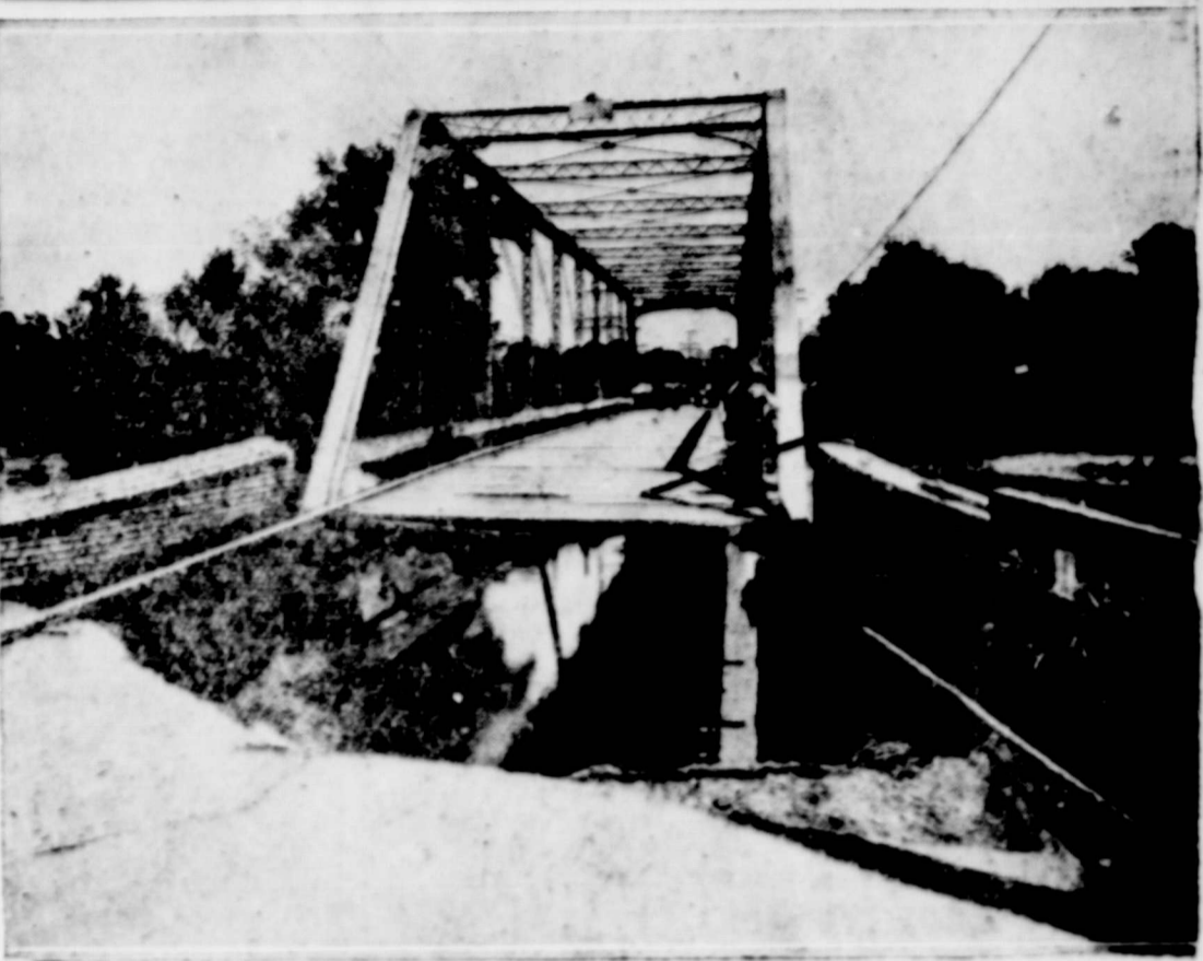
A storm which swept the central and southern part of Georgia of the past week resulted in thousands of dollars of damage to the highways and bridges. Above photo shows how approach to bridge on main highway running out of Macon was washed away. The damaged bridge over Walnut Creek resulted in a tie-up of traffic towards Augusta, Savannah and other central points.
