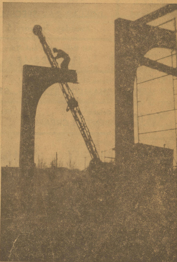
UP WITH FRAMEWORK—Structural steel framework of the new buildings for Friona's growing school goes up. Arrival of steel structural components of the building, which had delayed construction for more than a month, allows the Jones Construction crews to go ahead with erecting the school additions.
