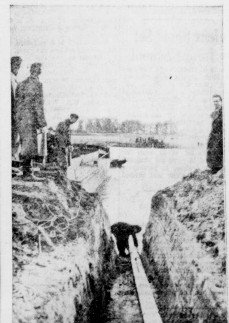
WELCOME ADDITION—A vital pipeline is laid between the Dutch villages of Oist and Welsum to carry a liquid as precious as any fuel. Made of plastic and measuring more than 480 feet, the pipeline extends under the River IJssel and provides drinking water for the villagers in the two towns.
