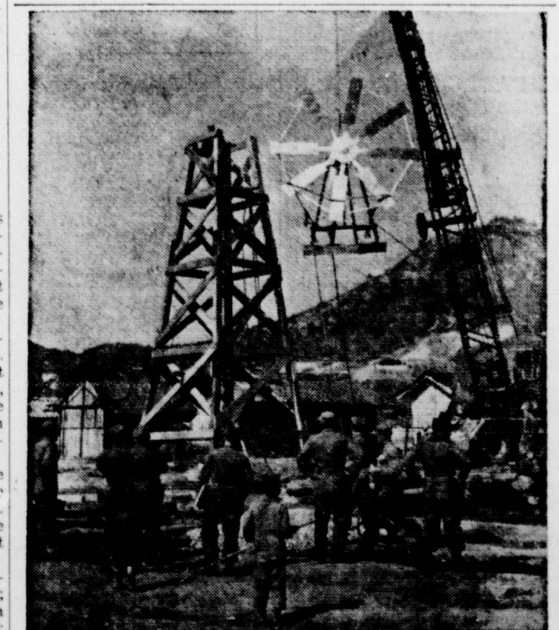
GOOD NEWS FOR KOREAN DON QUIXOTES is this windmill, first of its kind in the Land of the Morning Calm. The Third Engineer Combat Battalion of the U.S. Army's 24th Infantry Division built the structure to test practicability of pumping water by wind-power. Mrs. Syngman Rhee, wife of the President of the Republic of Korea, suggested the experiment, which appears to be successful.
