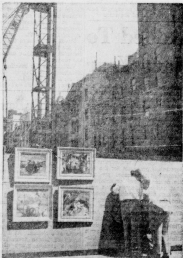
ART CAN WAIT—Some "sidewalk superintendents" are letting art take a back seat in New York. They're concentrating on the activity of a huge pile driver at work on the site of the old Brevoort Hotel, a Greenwich Village landmark demolished to make way for an apartment house. An outdoor art show was going on as these gentlemen seized their chance to peek.
