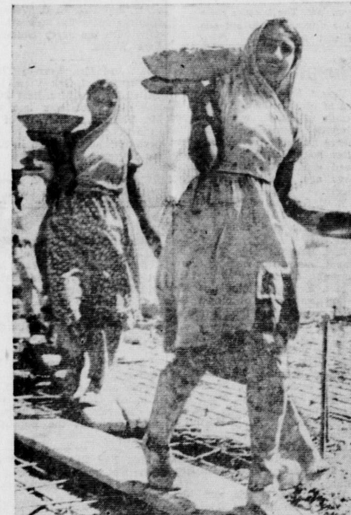
HELPMATES -These sturdy-limbed girls of Pakistan are not carrying cakes from ovens to sweethearts and husbands, but they are showing loyalty to their menfolk and their pride in their community. The "cakes" are trays of cement which are used in a building project that is designed to make Karachi a modern metropolis. The project is being jointly undertaken by the government and cooperatives to supply the residents with homes.
