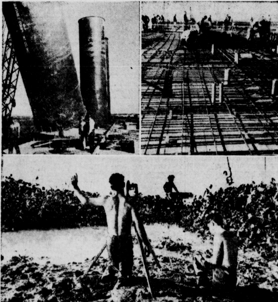
OPERATION SULPHUR —Huge flue gas heat reclaimers are swung into place at Garden Island Bay, La., to preheat millions of gallons of water for melting sulphur trapped in a salt dome beneath mud and water, upper left. The floor of the mining plant rises 16 feet above the level of the nearby Gulf of Mexico and workmen are laying steel reinforcing, right. A year ago, the area was desolation, but now a multi-million dollar plant is rising to tap a sulphur supply of untold value. Engineers stood hip deep in mud to survey it, below.
