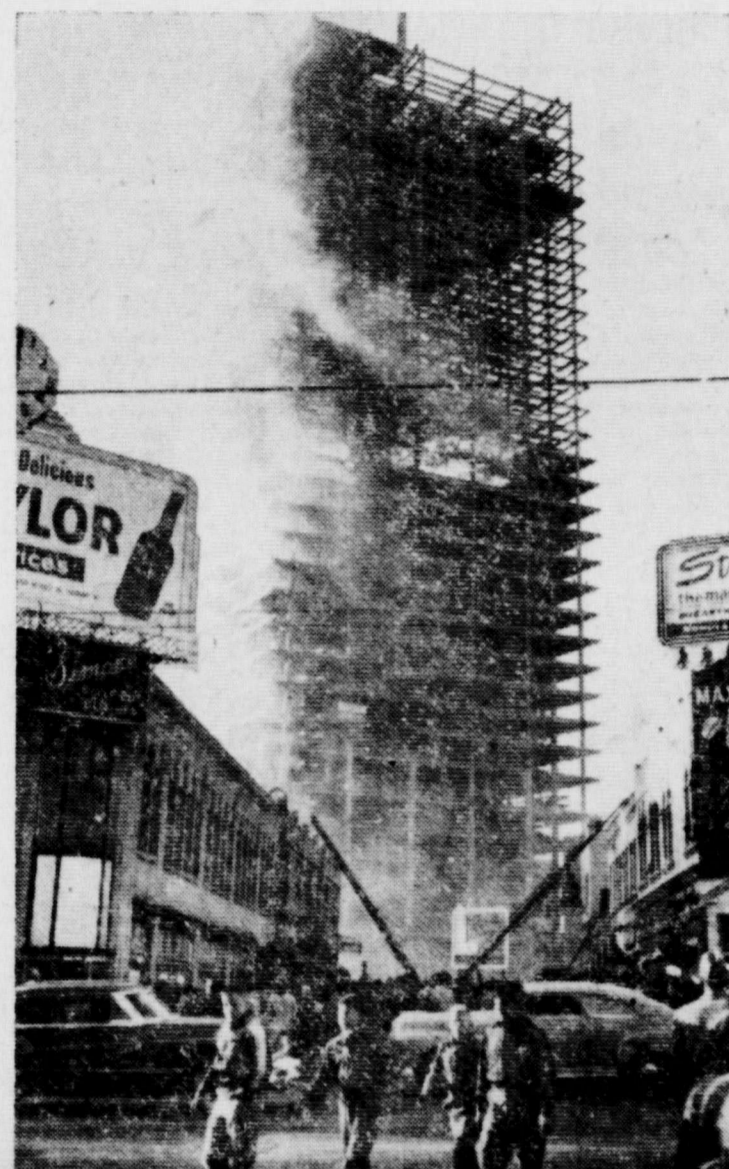
SKYSCRAPER FRAME AFIRE —Smoke sweeps through girders of the Republic National Bank Building under construction in Dallas, Tex., as firemen are called out to battle the four-alarm blaze. The fire started on the 20th floor and spread through five other floors before it was brought under control. Because of low water pressure, firemen had considerable difficulty.
