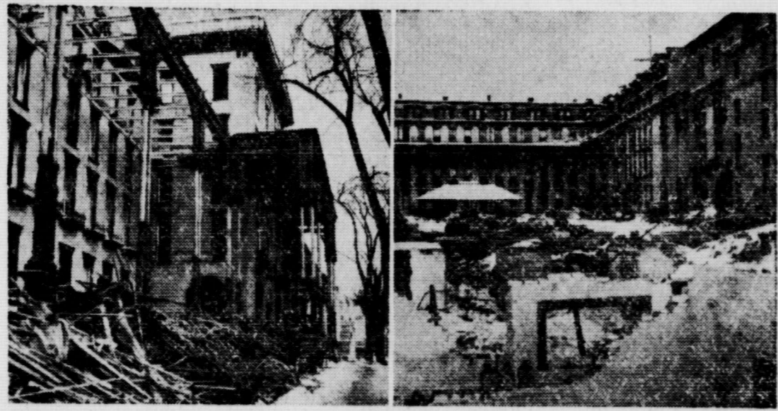
END OF A LANDMARK—The once-famed Grand Union Hotel in Saratoga Springs, N. Y., is surrounded with debris, left, as workmen raze the 150-year-old edifice to make way for a modern shopping center. Three old whiskey jugs, right, seem out of place during the proceedings.
