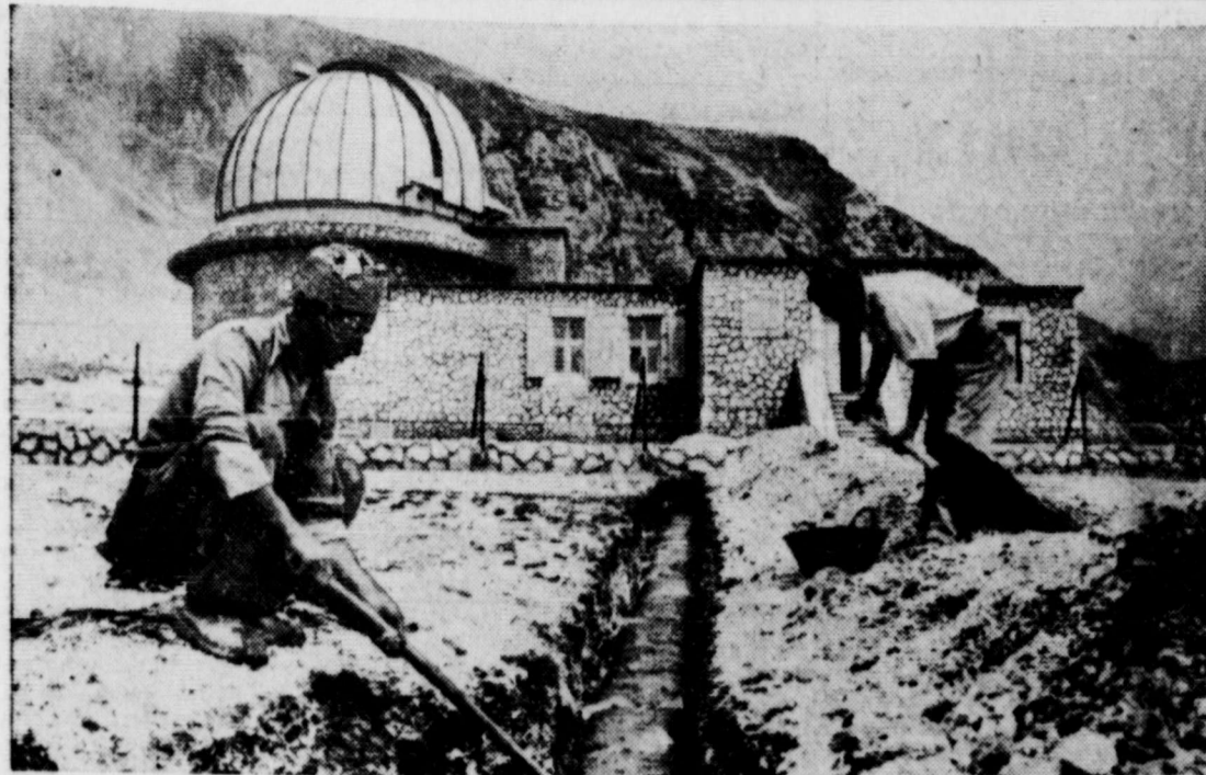
NOT FAR FROM ROME—Workers are putting finishing touches to the grounds of the new Gran Sasso Observatory which is in one of Italy's wildest mountain regions. It has the latest astronomical gear and powerful lenses, and is placed 6700 feet above sea level.
