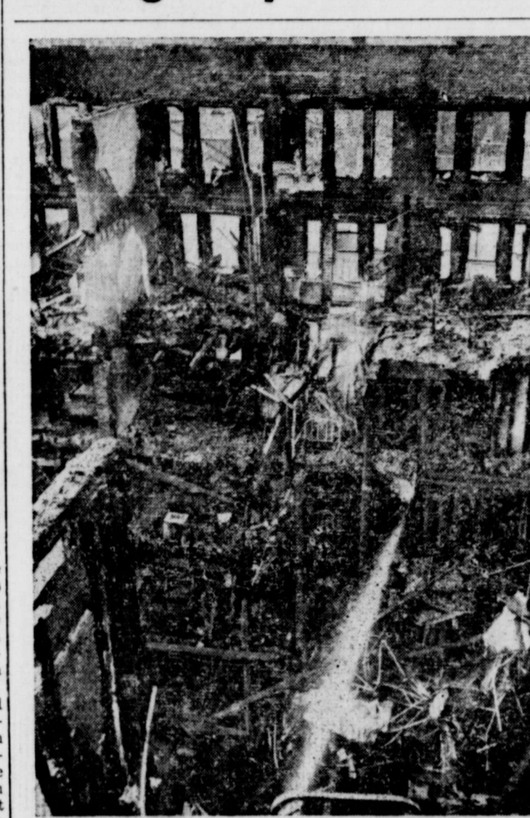
MILLION-DOLLAR ASHES—Scorched remains of a seven-story fire at a hotel in Philadelphia attest to the fierce flames that firemen battled through to rescue 150 guests from the seven-story building and million-dollar blaze. Sixteen firefighters were overcome by smoke, and more than a dozen guests, trapped on upper floors, were rescued on aerial ladders in the fire which was the city's largest in three years.
