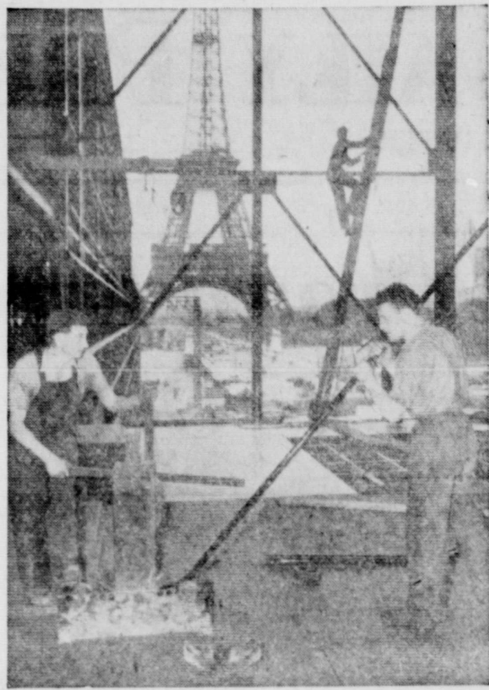
THEY HAVEN'T MUCH TIME—The Eiffel Tower provides the background in Paris as two French workmen twist tubing into the shapes needed to complete the United Nations Building in time for the General Assembly session to be held there in November. The dismountable building, attached to the Palais de Chaillot, will strike a new note in modern architecture.
