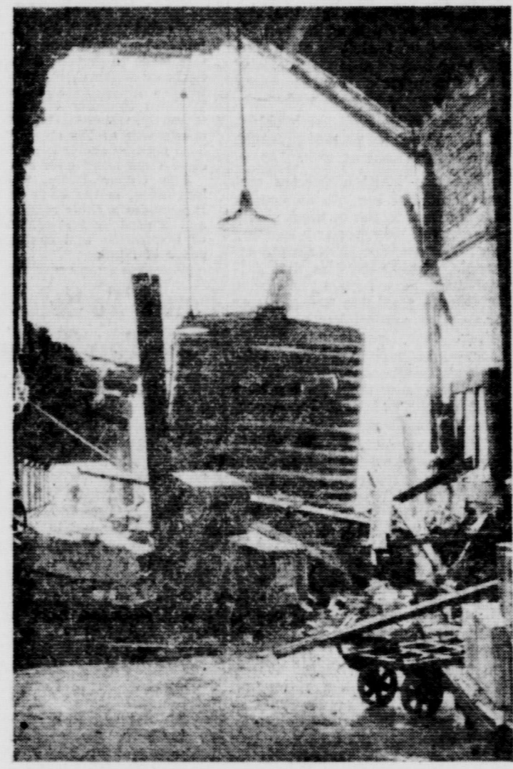
CLEAN THROUGH—This New York Central railroad freight car smashed a huge hole in the wall of a freight-house in Chicago, Ill., when it overshot the bumper guarding the wall. The car's wheels were stripped off but no one was injured in the accident.
