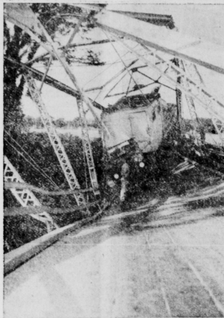
IT'S A REPEATER —A truck stands on a collapsed highway bridge near Shaw, Kans., after the span folded when the vehicle attempted a crossing. A few years ago, the opposite end of the bridge gave way under the weight of another vehicle.
