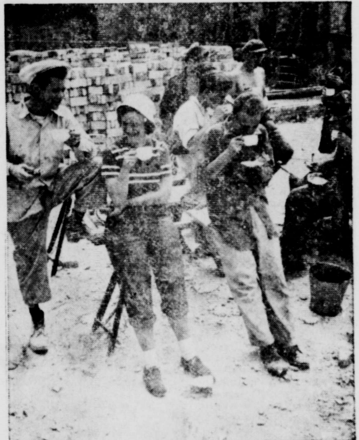
PITCHING IN—These students from the U. S., England, Holland, Switzerland, France, Denmark, West Berlin and from the Soviet zone, too, are helping to reconstruct Elizabeth Hospital in the British sector of Berlin. Work on the bomb-damaged building is being financed by the World Council of Churches.
