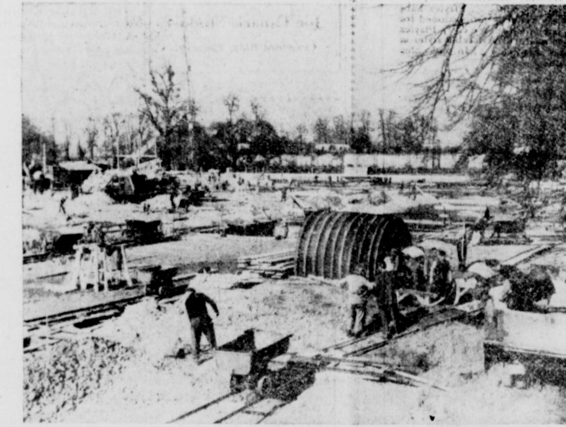
ENGAGED IN CONSTRUCTION—These are some of the 300 workmen engaged in the construction of the new building for the European Council in Strasbourg, France, which must be completed by the beginning of July. An inaugural ceremony officially started the building program.
