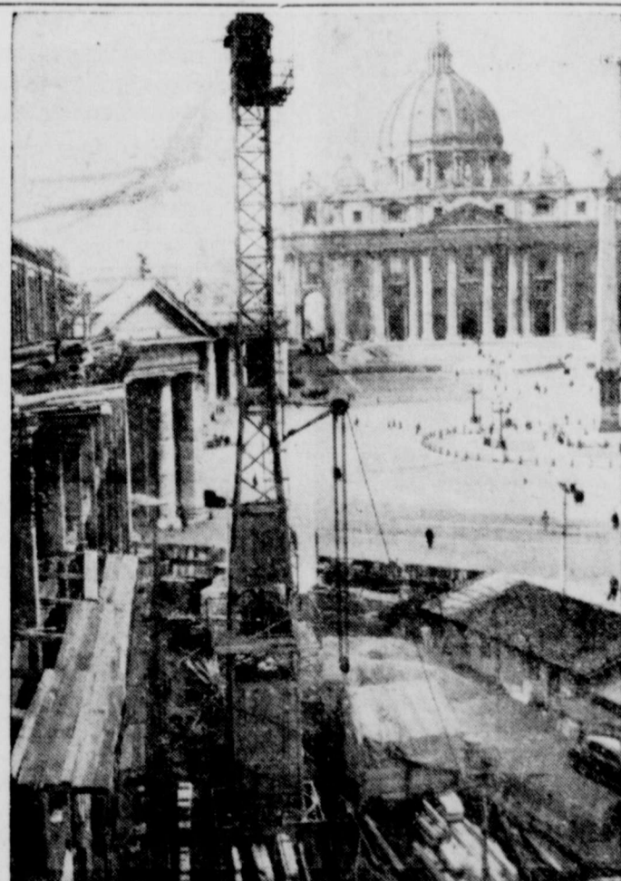
GETTING READY FOR THE RUSH —Rome, Italy, is getting ready for the pilgrims who will arrive to celebrate Holy Year. Two hotels, to accommodate 1200 pilgrims each, are being constructed at the end of the square facing the Basilica of St. Peter's and work on them should be completed in April.
