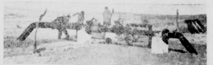
BEHIND YOUR GAS SERVICE there is something to build, paint, or repair every day—oftentimes in remote places. Above, a crew cleans up debris around control valves which are part of a new compressor station.
