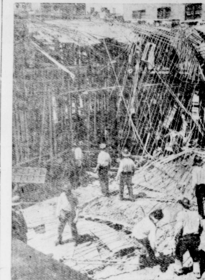
LOOKING FOR VICTIMS —A Bellevue Hospital disaster unit searches for injured in the reinforcing rods of a building which collapsed in New York. The flooring of the three-story building gave way unexpectedly and 20 workmen were hurt in the fall.
