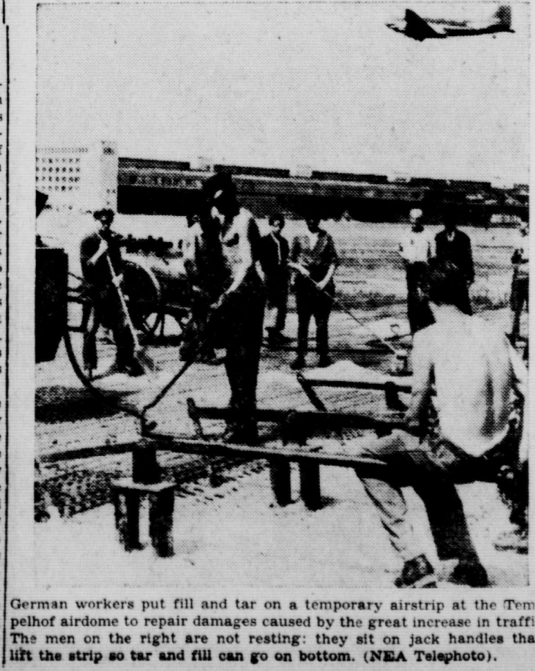
German workers put fill and tar on a temporary airstrip at the Tempelhof airdome to repair damages caused by the great increase in traffic.
