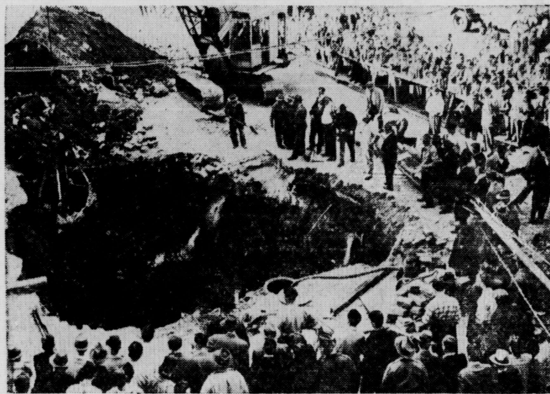
Emergency crews work in a desperate effort to extricate the body of Angelo Corsino, Chelsea, Mass., worker, that was buried by a cave-in. Spectators watch as a power shovel proved futile when sides of the 30 foot-square hole kept caving in and filling the excavation. (NEA Telephoto).
