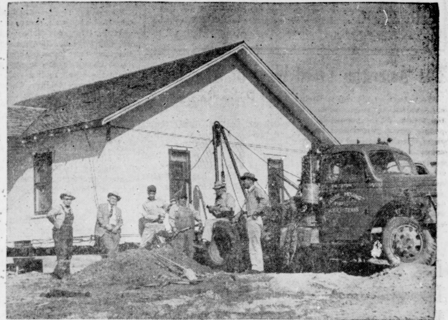
MOVING FOR RIGHT-OF-WAY —The M. R. Watkins' home, located two miles south of Meadow, was the first of nine houses to be moved off the Lubbock highway to make way for the new four-lane highway, to be constructed soon. Committeemen, appointed by the commissioner's court to secure the right-of-way, were on hand Tuesday of last week to oversee the project completed. All farmers and companies that have been contacted in regard to obtaining the necessary footage, have been agreeable to the requests, except for West Texas Cotton Oil Co., who has refused to oblige. Pictured in front of the Watkins' home, as it was being let down on the foundation, are Howard Guffin; Mack Thomason, committeeman; Gib Tatum; Cecil Chauncey; V. W. Johnson; and Jake Fulford, committeeman. (Staff Photo.)
