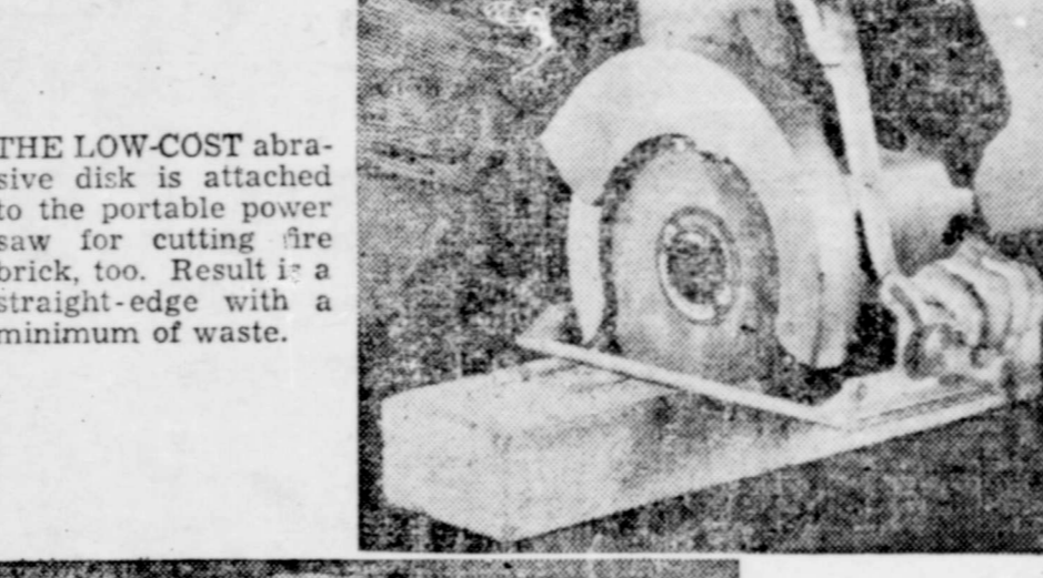
CUTTING a groove in concrete for installation of oil lines, left, takes only a few minutes with a power saw. An abrasive disk is used for this. Goggles should be worn.
