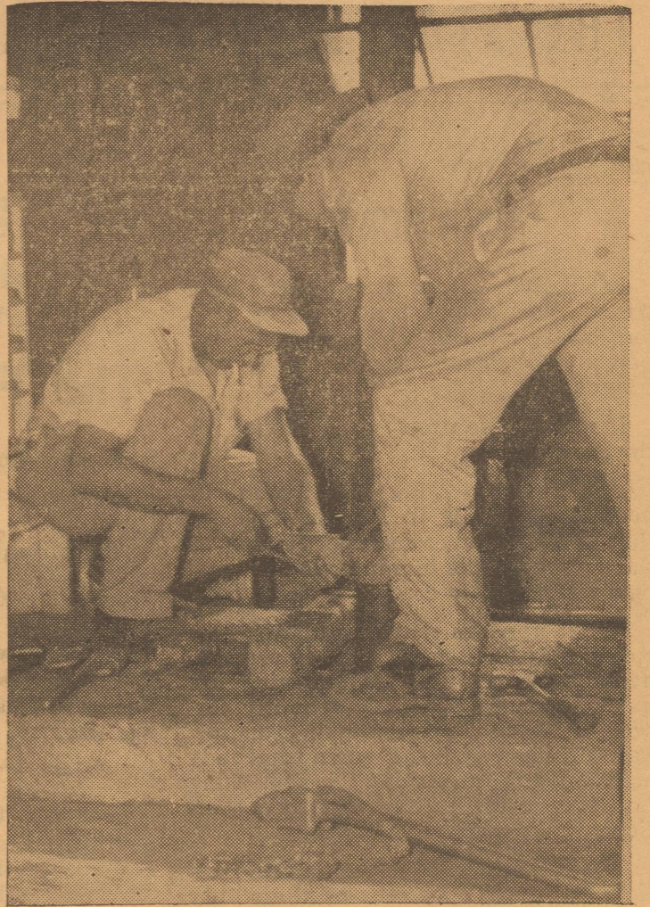
RUSTY PIPE FROM AN ONLY DAMP HOLE — City water department employee Clyde Fields and a pump service worker help with the "operation well doctoring," begun by the city as it looks for more water. Later the hole was bailed and chemical added to try and get water from the well that ran nearly dry about two weeks ago.
