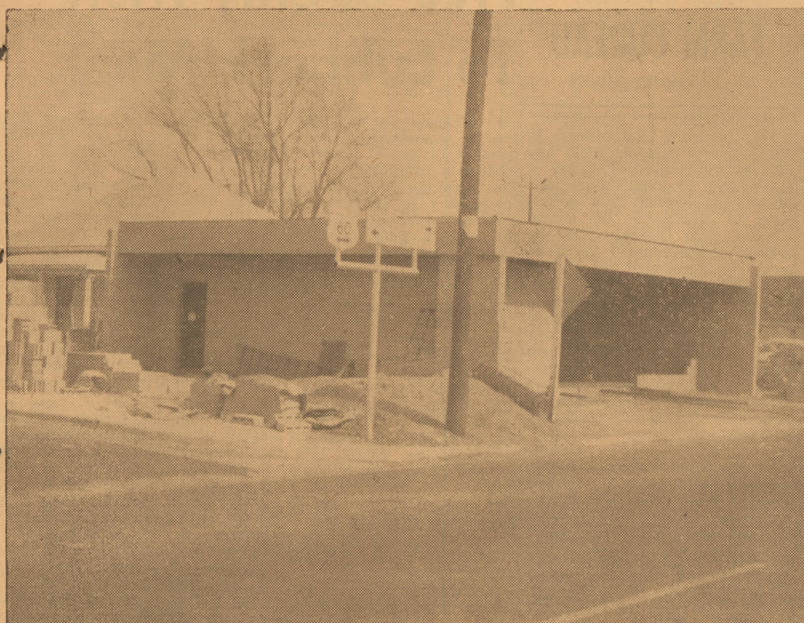
WON'T BE LONG NOW—This is the new Douglas-Bingham building going up at the intersection of Highway 60 and Main. Raymond Fleming, contractor, says cold weather is delaying work, but he still hopes for February completion.
