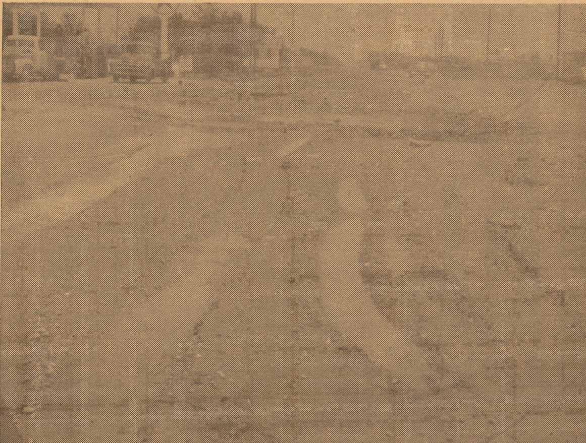
BOGGY THOROUGHFARE —This view of Highway 60 through Friona, which is undergoing extensive work as a part of its being widened to four lanes, would compare favorably with some of the old timers' pictures which show cars and wagons hub-deep in the mud of the 1920's. About two-thirds of the pavement was removed at this point, and traffic was forced to a narrow strip on the south side. Frequent showers which have fallen during the past three weeks have turned the scene into a quagmire.
