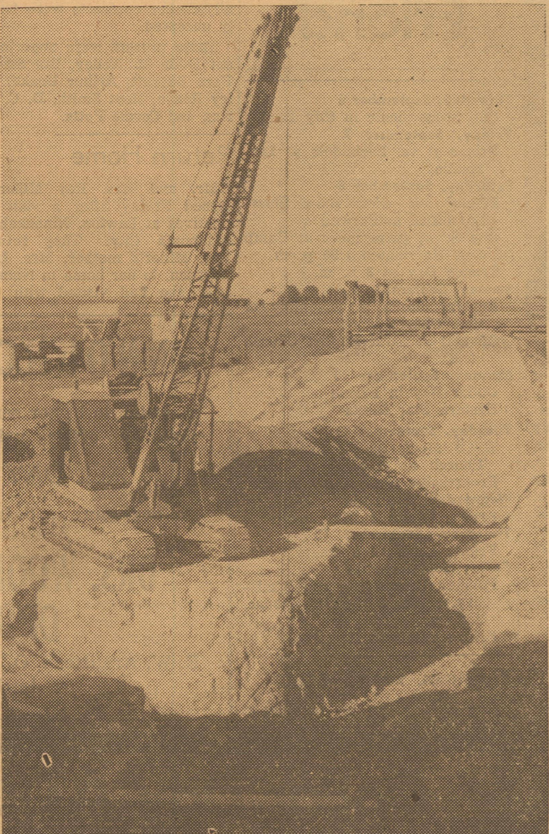
DOWN SHE GOES—It's a long way to the bottom of this excavation which will be under the new concrete elevator being built for Tri-County Elevator at Black. Monday was Labor Day, but it was no holiday for construction men at the scene, who are trying to finish the job in time for harvest.
