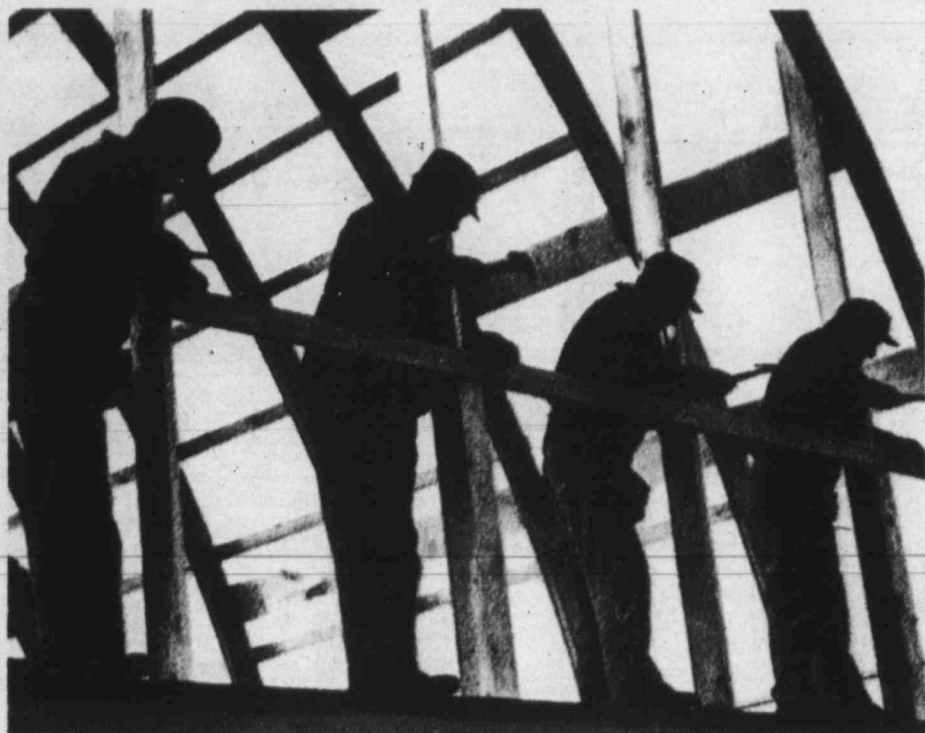
ALL TOGETHER, NOW — Hammers are swinging in unison as Marshfield, Wis., area farmers nail together at an old-fashioned barn raising on the Alfred Thompson farm. Thompson's neighbors are helping replace another barn that burned to the ground last month. The farmers are, left to right, Duane Guden, Roger Heeg, Arthur Guden and James Reno.
