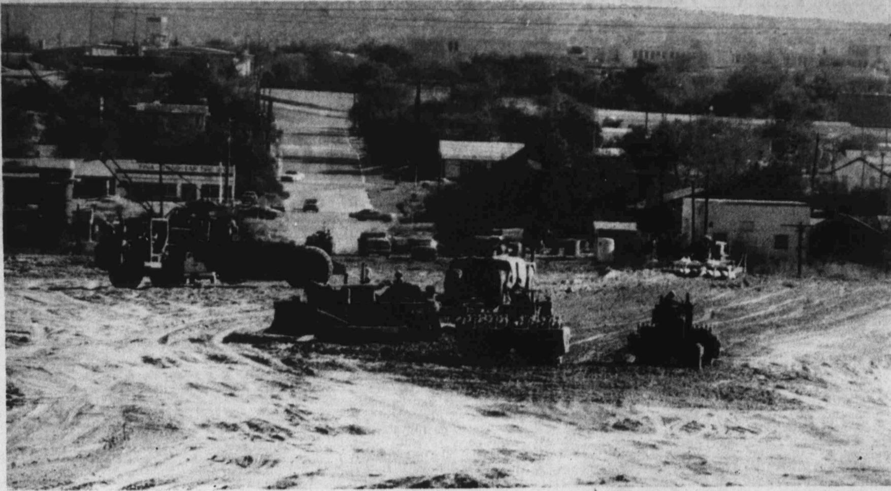
TO BECOME A REALITY — The long sought Owen Street overpass is actually under construction with land being cleared at the site and groundwork underway. This is a view looking south, with Big Spring High School shown on the rise off to the right of the photo.
