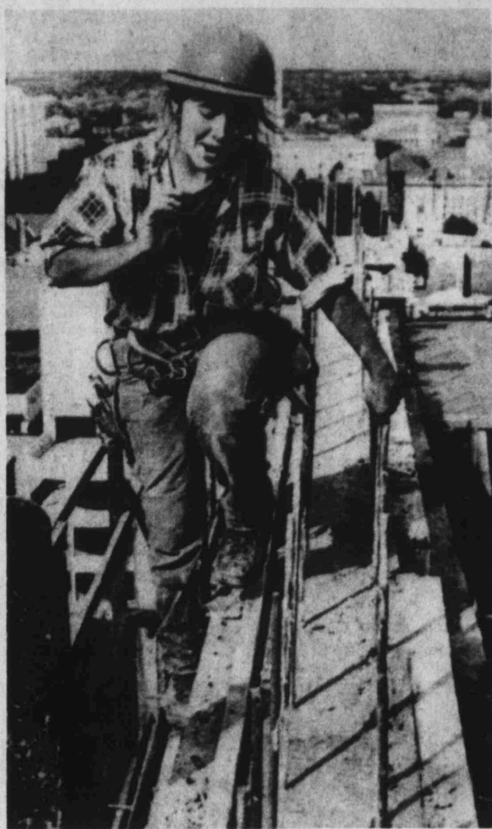
REAL LIFT — Cynthia Slade, 21, a second year carpenter's apprentice, says her work atop a 160 foot tall bank building "gives me a real lift."
